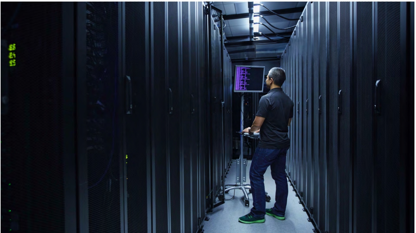
Optimizing data center energy efficiency is crucial
